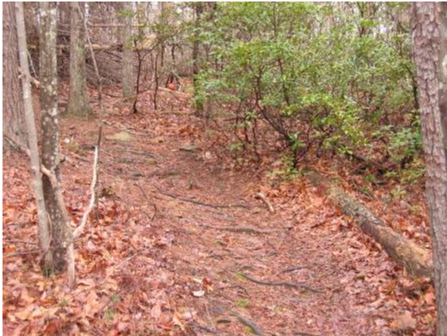
This is another view of the same unsustainable section, too steep, for too long. Water based erosion has exposed many roots, causing users to widen the trail by selecting more walkable and rideable lines.
