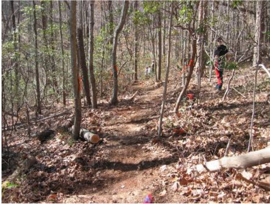
View of the reroute while under construction. The reroute uses a sustainable grade, going across a side slope, and it has grade reversal features for drainage.
